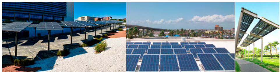
Figure 8. Sample installations shown on APS Website. Source: APS ( http://www.apowersolutions.com/ )
