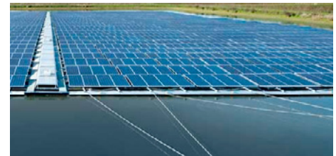
Figure 2. Floatovoltaics by SPG.
